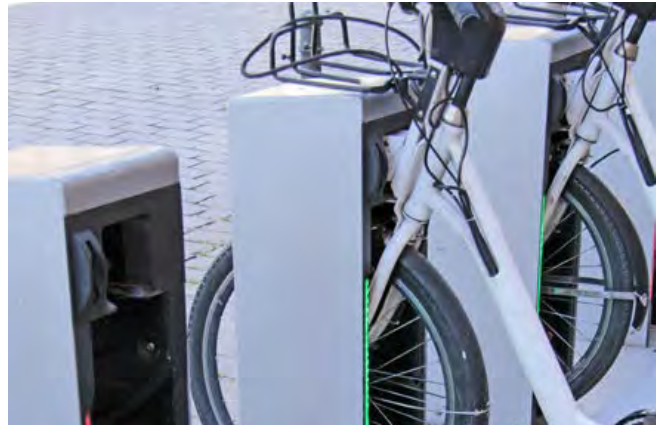
E-Bike Charging Stations support emission free transportation to, from, and within Comox parks and trails.
