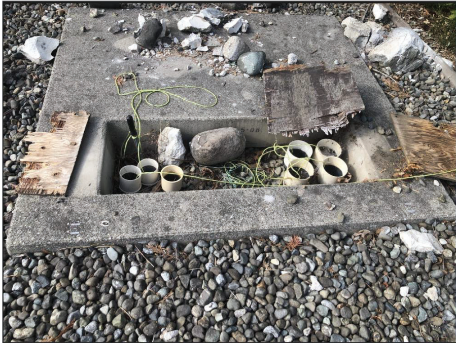
Photo 5 – Open wells at the southeast perimeter of the Site.
