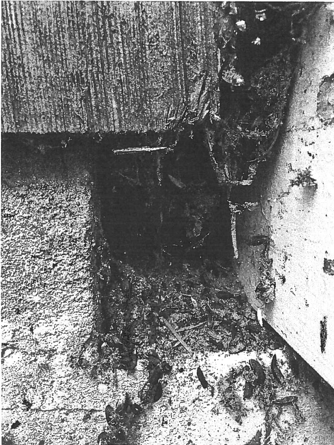
Termite damage in basement sill.
