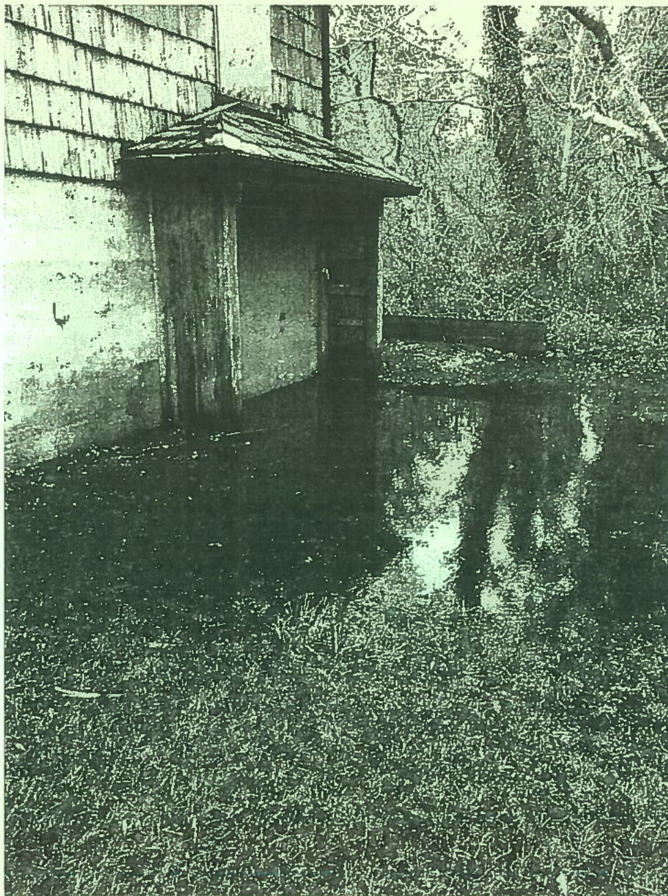
March 07/2016. This was caused by rainfall only.
