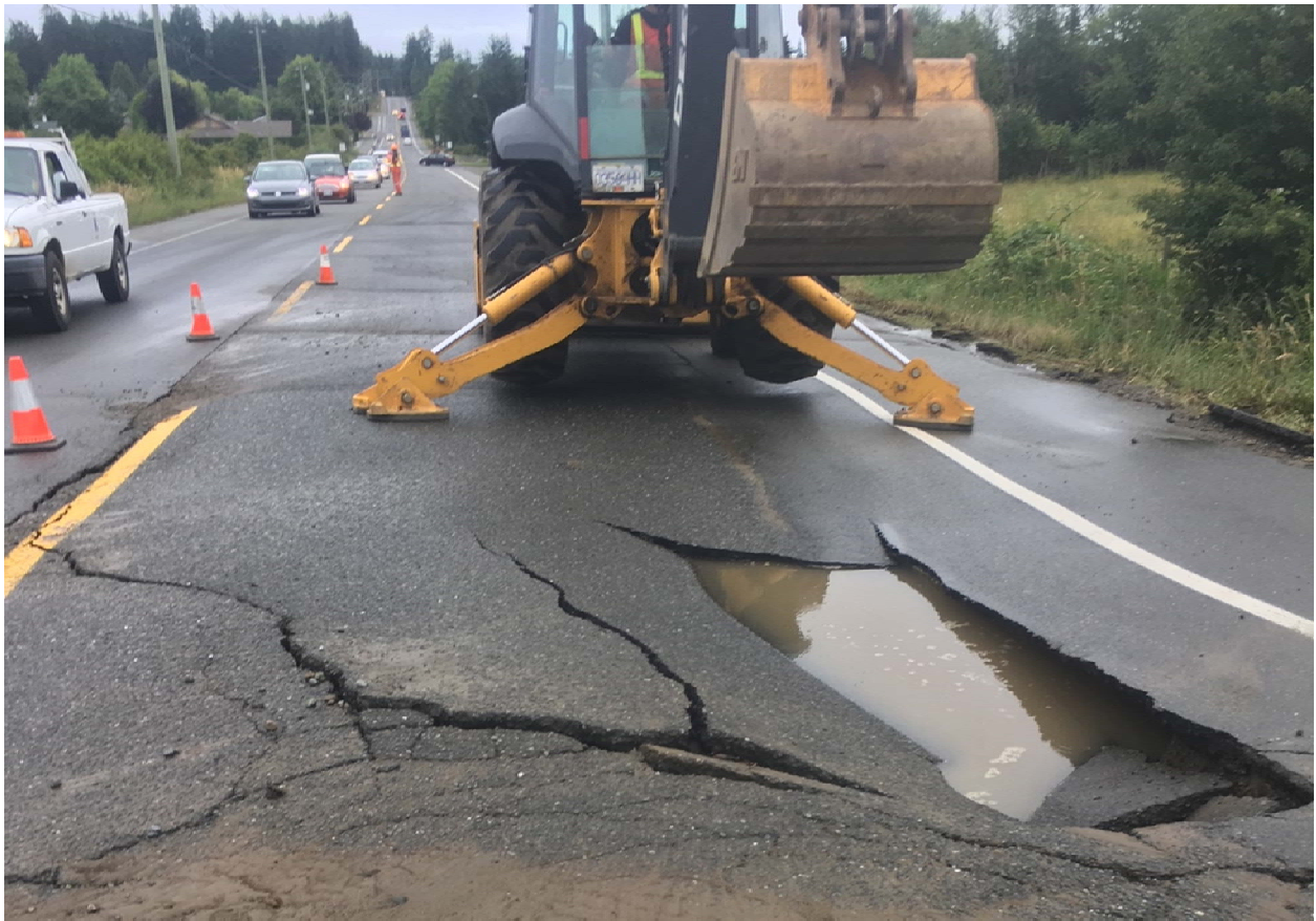
Guthrie Road water main break
