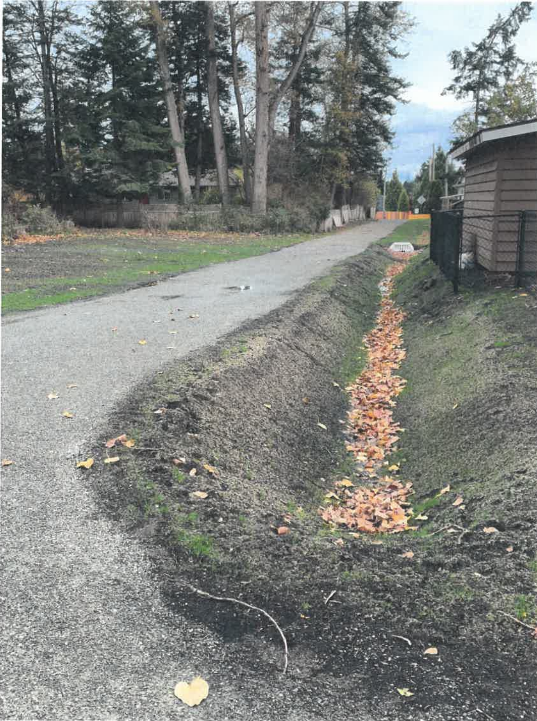
McLeod St to Douglas St Water and Storm Upgrade – Looking east from McLeod end of pathway.
